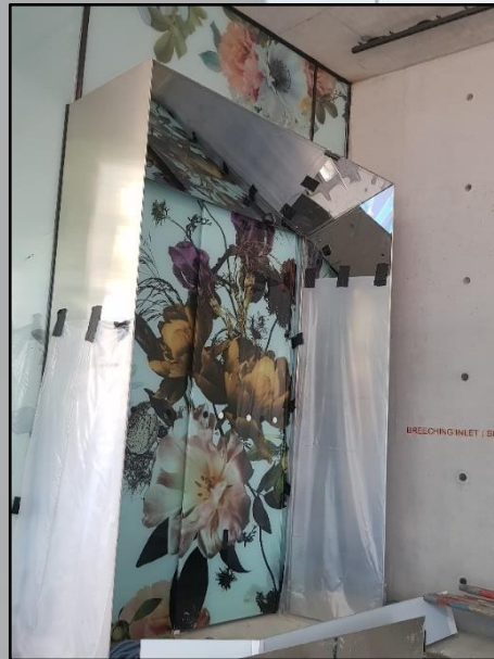
Auto-Sliding Glass Door with SS Portal @ Entrance
